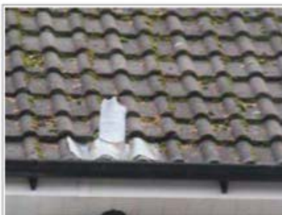
Missing vent pipe
