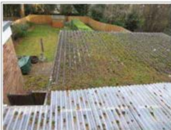
Mossy garage roof
