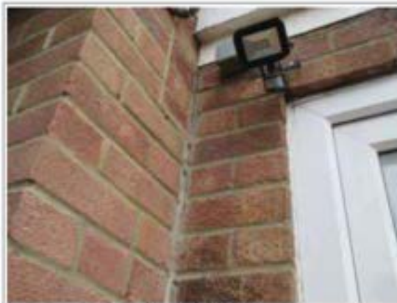
Crack at junction
